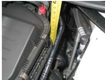
It is seven inches below the driver side rear corner of the airbox.
